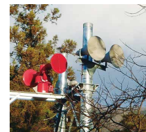
Water release alarm station
