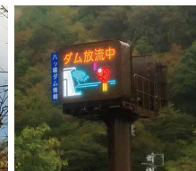
Water release alarm display equipment
