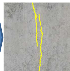
[ひび割れA自動検出]
