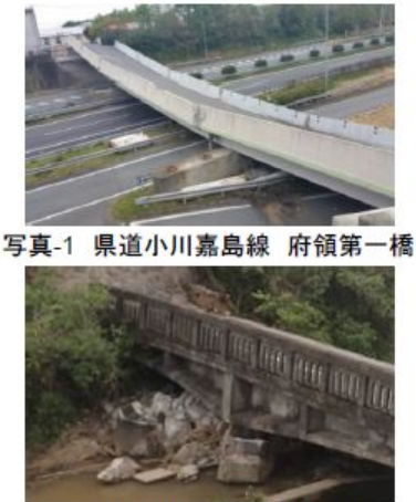
写真-2 平田・小柳線 田中橋: A photograph showing a bridge structure with significant damage to the concrete railing and support.
