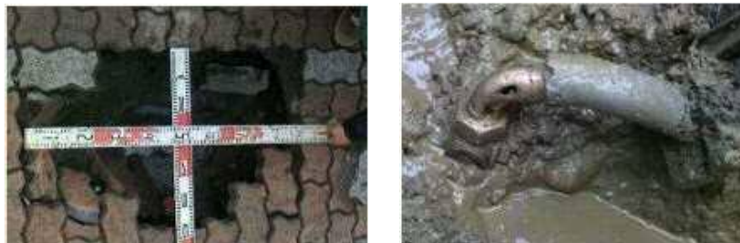
路面陥没 約0.6m×0.9m×0.35m(深さ)
