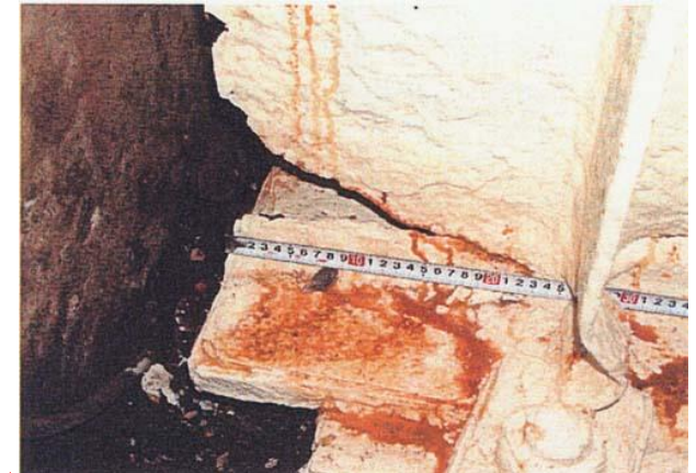
断面欠損と座屈
