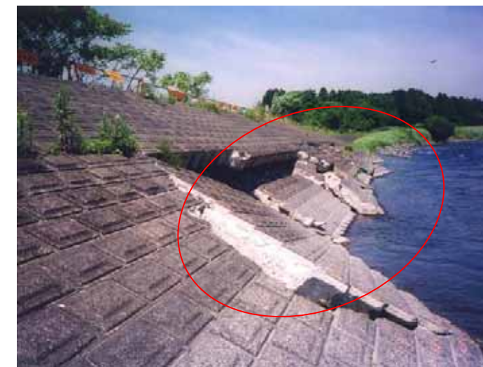
護岸の洗掘・崩
