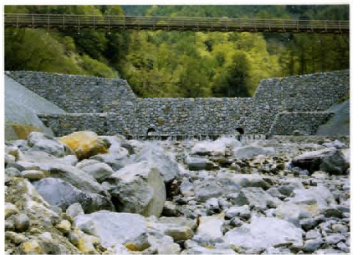
⑫ 石室川第六砂防えん堤 Ishitorogawa No.6 Sabo dam 構造物表面に河床の巨石を積み、景観に配慮した砂防えん堤。 This sabo dam has actual river stones on the structure surface for environmental concerns.
