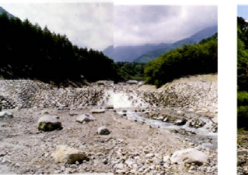
⑭ 青木床固群 Aoki groundfills 現地発生巨石を型枠替わりとし、コスト削減を図り、なおかつ現地環境に合うよう整備および計画されている床固群。 This facility is being prepared and planned by utilizing the locally found stones as the formwork for cost reduction as well as for local environment concerns.
