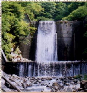
45 中島砂防えん堤 Nakajima dam 釜無川上流域で最も高い大規模砂防えん堤 The tallest huge Sabo dam in the Kamanashi river upper reaches
