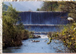
16 絡窟砂防えん堤 Mulinakutsu dam 釜無渓谷の出口を守る砂防えん堤 Sabo dam securing Kamanashi valley end
