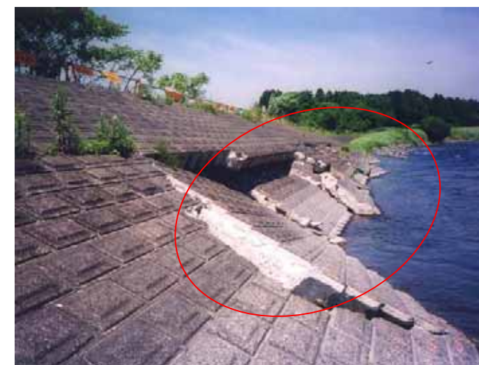
護岸の洗掘・崩
